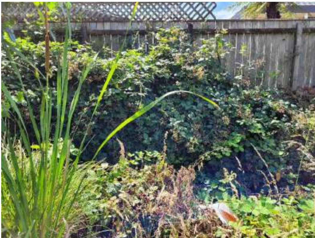
Photo 8: Likely location of existing western culvert. Not sighted due to dense vegetation.
