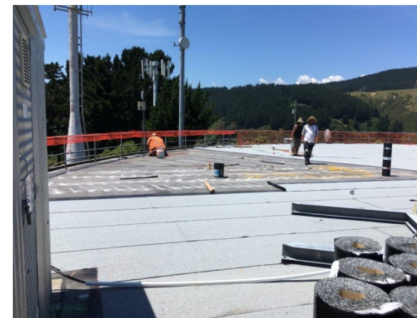
Application of a specialist coating to seal the roof of the Riwai water supply reservoir
