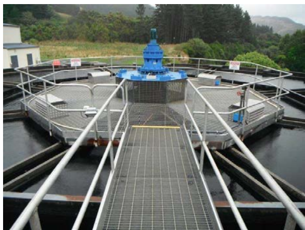
The clarifier at the Waikanae water treatment plant showing the central mixing area and surrounding settlement areas
