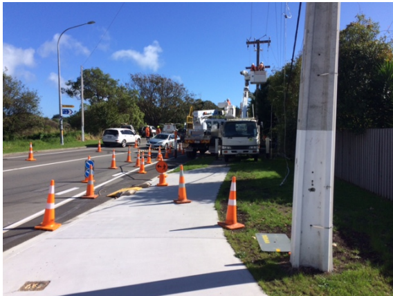
Undergrounding of overhead services on Te Moana Road before footpath widening can proceed
