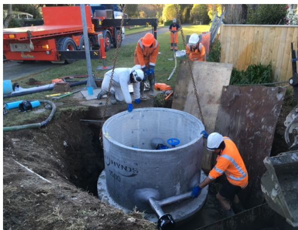
A new, pre-assembled valve chamber being installed at the Puriri Road wastewater pumping station
