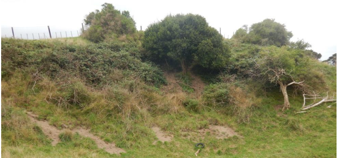
Figure 22. Photograph of the hillside along the northern boundary of 65 Ratanui Road, looking northwest
