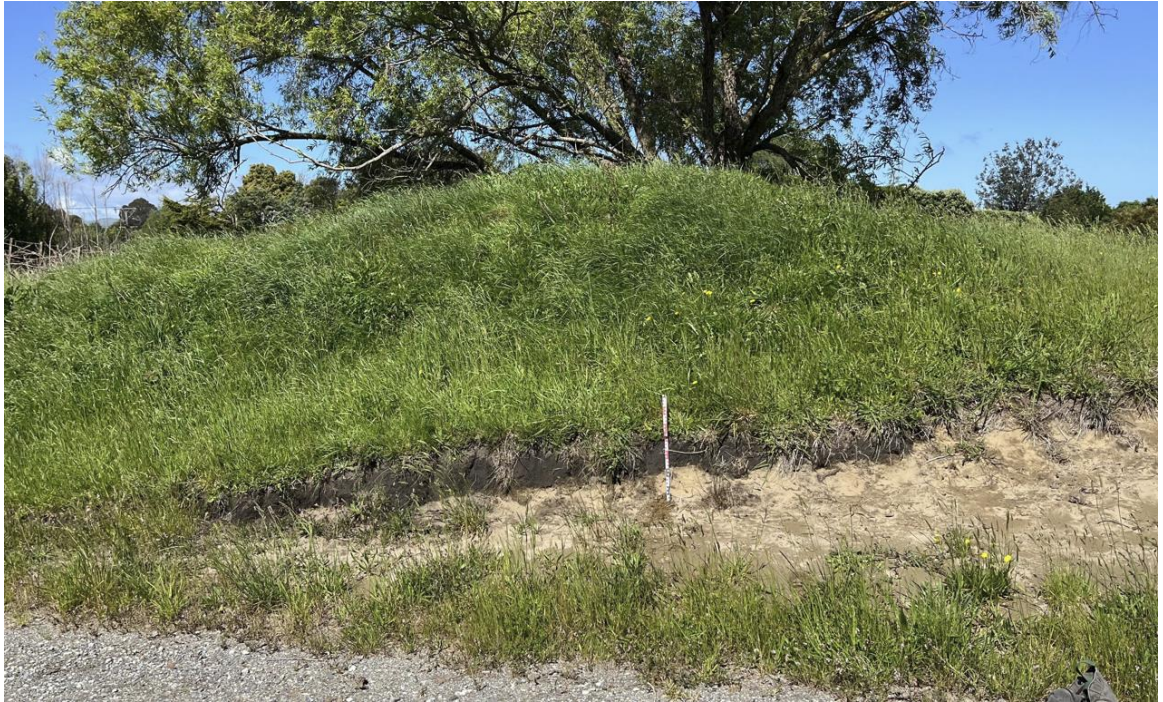
Figure 35. Photograph showing the cut profile alongside the track leading to Ratanui Road, looking west (1m scale)
