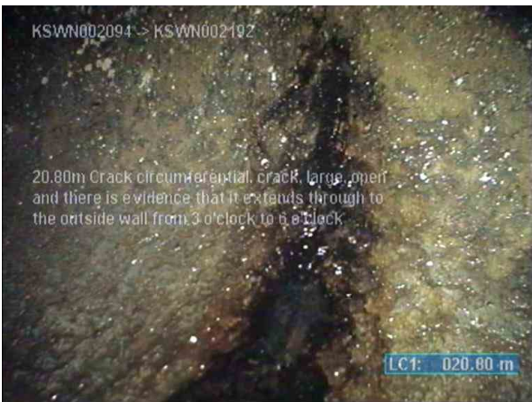
KSWP003817_db4cbf4f-896b-4697-8544-55b7a58b3b42_20220812_113238_708.jpg, 00:04:32, 20.80m (35.20m) Crack circumferential, crack, large, open and there is evidence that it extends through to the outside wall from 3 o'clock to 6 o'clock
