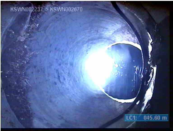
KSWP003713_4a77d837-2bba-4c40-a44b-a017512c4149_20220811_132102_186.jpg, 00:04:31, 45.60m (2.60m) Gap separation width 20mm
