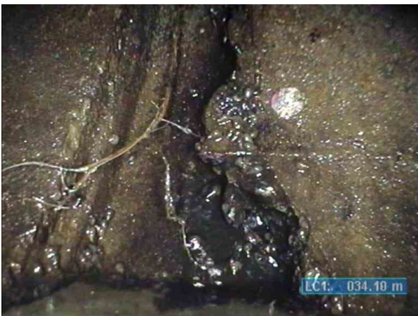
KSWP003817_700bbb4a-d05f-4d20-bcb1-caed32b5e03b_20220812_113613_212.jpg, 00:07:24, 34.10m (21.90m) Joint damaged/chipped, large, clearly through the pipe wall from 3 o'clock to 9 o'clock / Infiltration and broken
