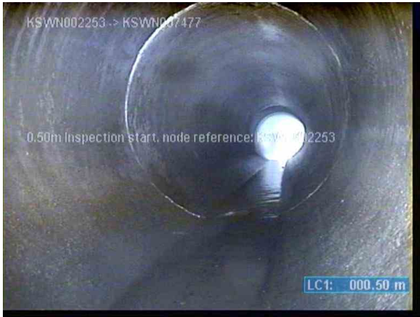
KSWP003634_1ba1942e-786e-4d32-a0ef-3e5e99191770_20220708_155106_788.jpg, 00:00:18, 0.50m Inspection start, node reference: KSWN002253
