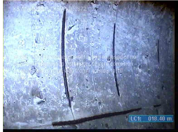
KSWP004512_0244a32f-c0b6-44dc-be00-d1b417667dd6_20220711_125619_066.jpg, 00:02:44, 18.40m Surface damage, reinforcing exposed or no longer present due to corrosion, severe corrosion or deep voids in pipe wall from 7 o'clock to 10 o'clock
