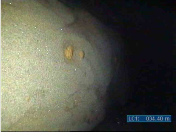
KSWP003817_87ccedcd-31e1-4b81-b037-d14fae2386ca_20220812_113645_304.jpg, 00:07:47, 34.40m (21.60m) Debris silt, small, clear diameter reduced by less than 10%, start
