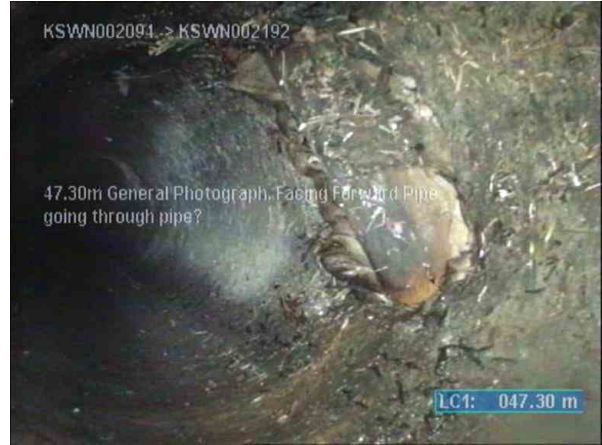
KSWP003817_571327f2-f20b-48b4-873b-7e7518a073fb_20220812_113946_888.jpg, 00:10:25, 47.30m (8.70m) General Photograph, Facing Forward / Pipe going through pipe?
