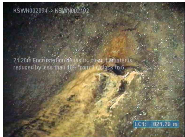
KSWP003817_c9bedc18-acc9-4587-be8a-7ff7d5d63b6e_20220812_113306_569.jpg, 00:04:55, 21.20m (34.80m) Encrustation deposits, clear diameter is reduced by less than 10% from 3 o'clock to 6 o'clock
