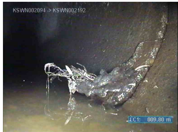
KSWP003817_35b78b62-6938-4352-9f91-7300c8ca4902_20220812_113006_929.jpg, 00:02:18, 9.80m (46.20m) Joint damaged/chipped, large, clearly through the pipe wall from 4 o'clock to 6 o'clock / Roots
