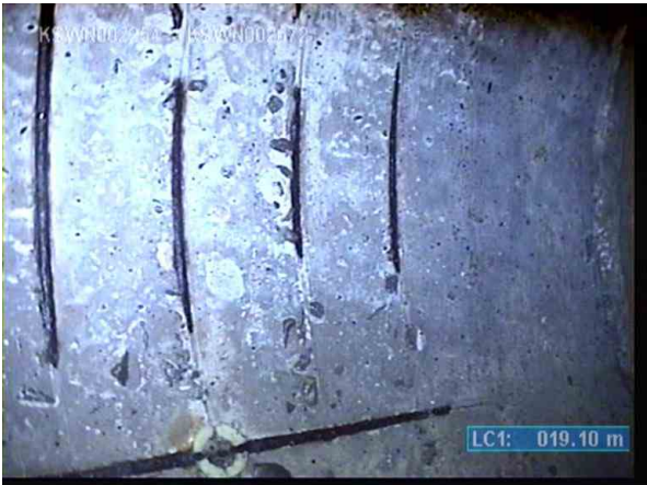
KSWP004512_060d03ac-41e2-4c53-bf61-835357fe24d4_20220711_125640_322.jpg, 00:03:03, 19.10m Surface damage, reinforcing exposed or no longer present due to corrosion, severe corrosion or deep voids in pipe wall from 7 o'clock to 10 o'clock
