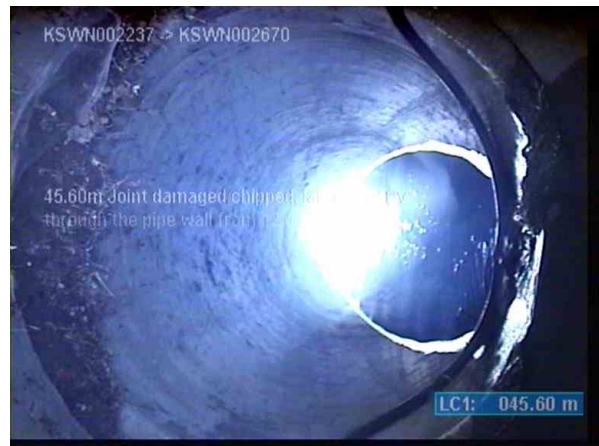
KSWP003713_bdd97187-9c4c-4e12-97c5-650296e93888_20220811_132048_371.jpg, 00:04:25, 45.60m (2.60m) Joint damaged/chipped, large, clearly through the pipe wall from 12 o'clock to 12 o'clock
