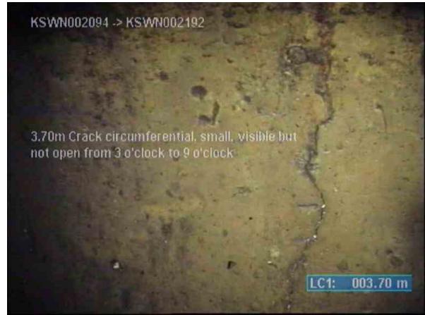
KSWP003817_06475611-4031-46c4-9258-8a08b54254d5_20220812_112909_255.jpg, 00:01:29, 3.70m (52.30m) Crack circumferential, small, visible but not open from 3 o'clock to 9 o'clock
