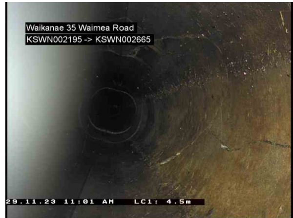
42_KSWP003751_200.jpg, 00:03:25, 4.50m (10.90m) Cracks multiple, medium, crack open but there is no evidence that the crack extends to the outside wall from 10 o'clock to 3 o'clock
