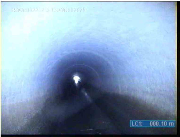
KSWP003713_8fcaed6d-e316-4503-bd38-4c2f453a4dee_20220811_131533_459.jpg, 00:00:10, 0.10m (48.10m) Inspection start, node reference: KSWN002237
