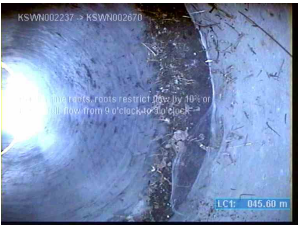
KSWP003713_90419e6e-c99a-4298-a253-86fee32cceed_20220811_132134_875.jpg, 00:04:52, 45.60m (2.60m) Fine roots, roots restrict flow by 10% or less of full flow from 9 o'clock to 3 o'clock
