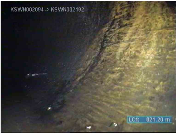
KSWP003817_0914ca62-fff3-4eec-9a37-9975186a6ff3_20220812_113311_329.jpg, 00:04:55, 21.20m (34.80m) Encrustation deposits, clear diameter is reduced by less than 10% from 3 o'clock to 6 o'clock
