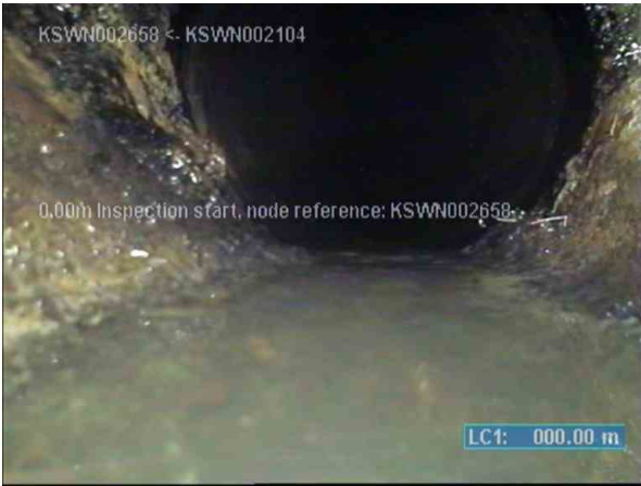
KSWP004528_e003fdb0-c8ea-45e4-96ca-35ff473e65db_20220809_111906_286.jpg, 00:00:12, 0.00m (48.70m) Inspection start, node reference: KSWN002658
