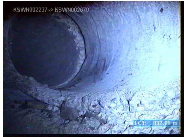
KSWP003713_ba39b8cc-c631-4d6d-bf67-e948ee438793_20220811_131924_634.jpg, 00:03:14, 32.80m (15.40m) The lateral is open at 9 o'clock / Ok
