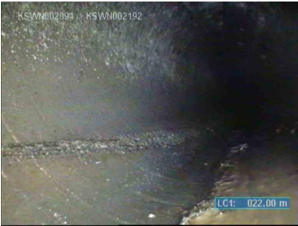
KSWP003817_af5911e6-1802-49a9-9655-90a61d5d830e_20220812_113403_886.jpg, 00:05:30, 22.00m (34.00m) Fine roots, roots restrict flow by 10% or less of full flow at 9 o'clock
