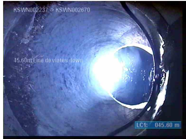
KSWP003713_71c9edd4-90be-4488-97db-24646cada9ca_20220811_132110_921.jpg, 00:04:37, 45.60m (2.60m) Line deviates down
