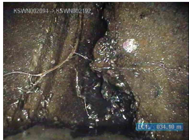
KSWP003817_adfc3087-874e-45aa-86b4-190dc5edbc04_20220812_113624_055.jpg, 00:07:30, 34.10m (21.90m) Infiltration, running (visibly moving) flow from 3 o'clock to 6 o'clock
