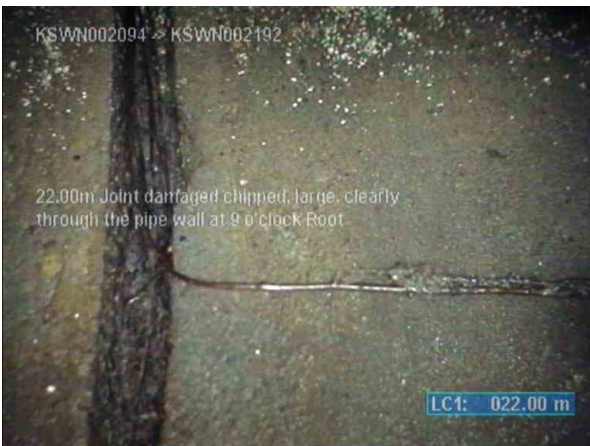
KSWP003817_bf9a678e-ebf6-4e9e-a17c-8ff011637ce3_20220812_113348_222.jpg, 00:05:24, 22.00m (34.00m) Joint damaged/chipped, large, clearly through the pipe wall at 9 o'clock / Root
