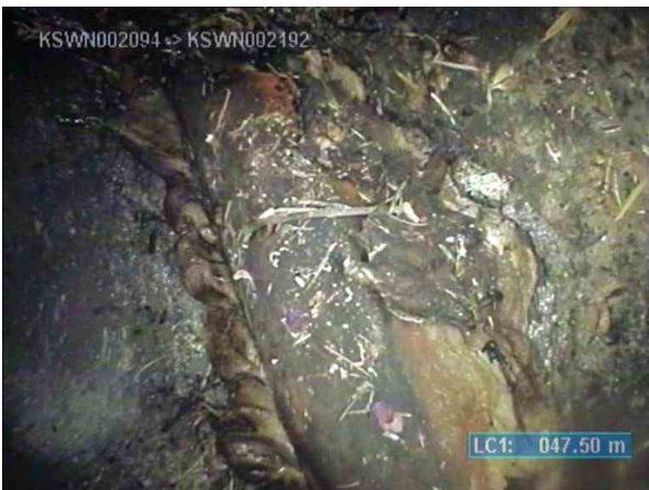
KSWP003817_7ca395ac-03b1-4232-b42e-49f3617e2889_20220812_113954_174.jpg, 00:10:25, 47.30m (8.70m) General Photograph, Facing Forward / Pipe going through pipe?
