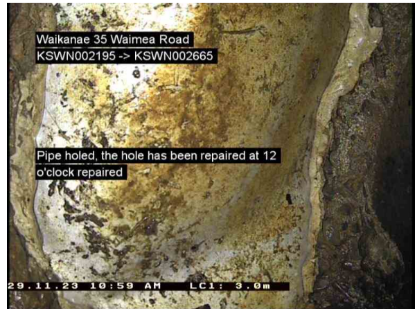
42_KSWP003751_196.jpg, 00:02:26, 3.00m (12.40m) Pipe holed, the hole has been repaired at 12 o'clock / repaired
