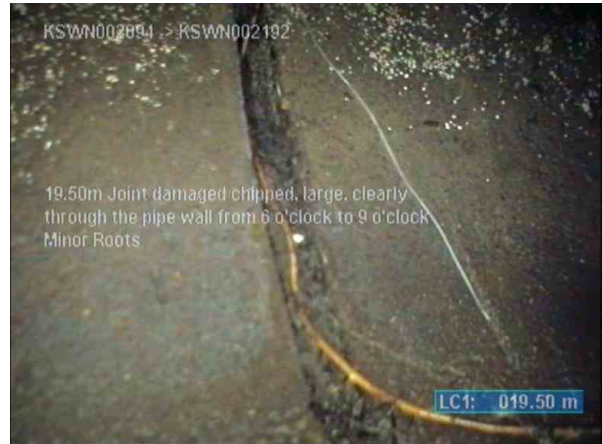
KSWP003817_36c32fb4-a4dc-41d3-aa9c-aab22b83395a_20220812_113157_910.jpg, 00:03:54, 19.50m (36.50m) Joint damaged/chipped, large, clearly through the pipe wall from 6 o'clock to 9 o'clock / Minor Roots
