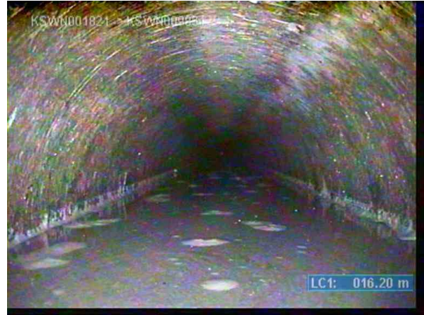
KSWP003815_6490fce0-0345-4d25-ac2c-1e2e453b3bc3_20220701_135213_247.jpg, 00:03:52, 16.20m General comment / High water level going to creek
