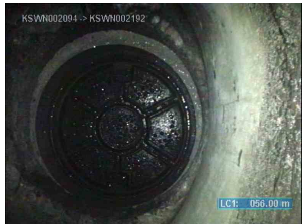
KSWP003817_a4fb2681-563a-48bd-83bd-c1cc76266e3d_20220812_114139_453.jpg, 00:12:14, 56.00m (0.00m) Inspection ends, node reference: KSWN002192
