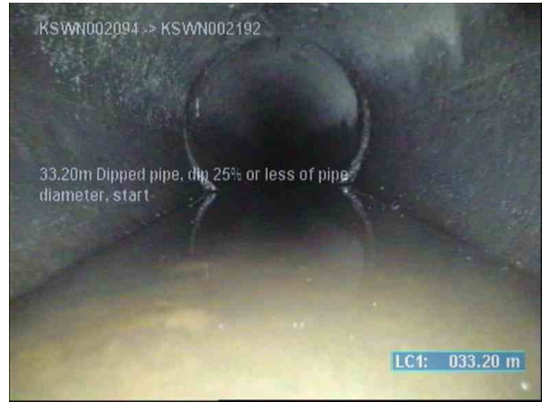
KSWP003817_c346b211-c8d1-4778-881d-df197c90eed6_20220812_113525_551.jpg, 00:06:53, 33.20m (22.80m) Dipped pipe, dip 25% or less of pipe diameter, start
