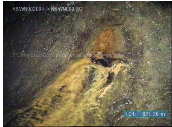
KSWP003817_17864e24-11e9-4cd5-acf6-a256721788ba_20220812_113319_750.jpg, 00:05:04, 21.20m (34.80m) Crack circumferential, crack, large, open and there is evidence that it extends through to the outside wall from 3 o'clock to 6 o'clock
