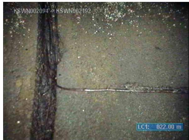
KSWP003817_da90fc7a-621a-40ac-8dd4-68883b6b4d57_20220812_113358_896.jpg, 00:05:30, 22.00m (34.00m) Fine roots, roots restrict flow by 10% or less of full flow at 9 o'clock
