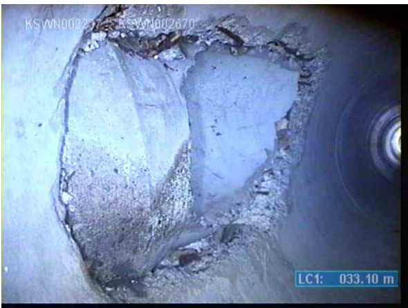
KSWP003713_ab94fea7-9b65-4da0-ae52-e7a3c67fc7da_20220811_131941_203.jpg, 00:03:14, 32.80m (15.40m) The lateral is open at 9 o'clock / Ok
