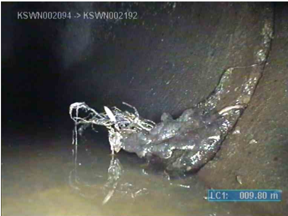
KSWP003817_c21fe9cd-398c-42ed-b7fb-1d5d78366c5d_20220812_113017_759.jpg, 00:02:25, 9.80m (46.20m) Fine roots, roots restrict flow by 10% or less of full flow from 4 o'clock to 6 o'clock
