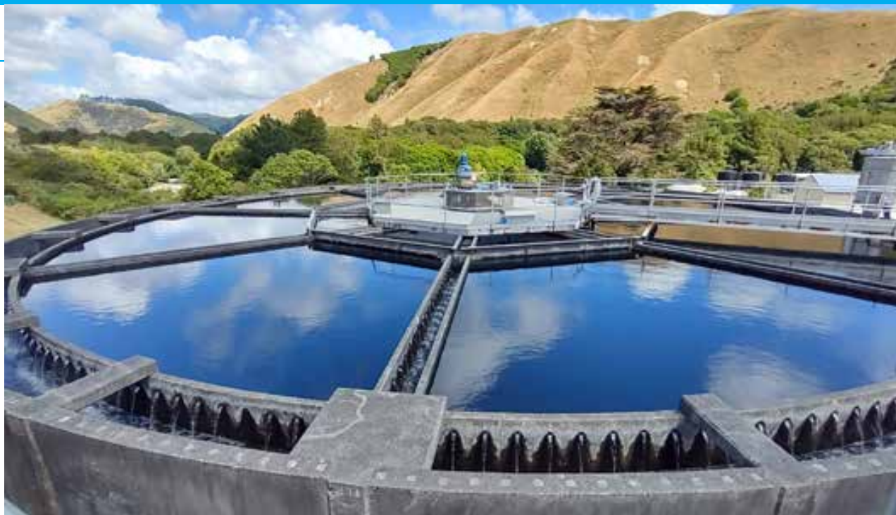
Waikanae water treatment plant.
