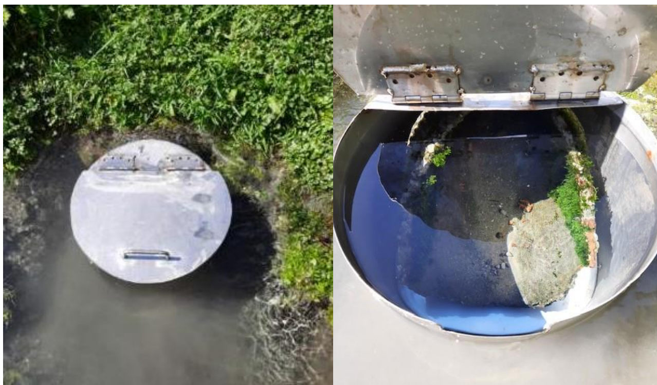
Figure 2-13 Installed Spring Sample Pot
