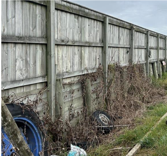
Figure 12. Existing fence and retaining between No. 160 Mazengarb Road and the Niu Sila Way properties
